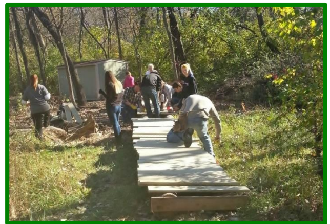
Workdays are a critical part of how important improvements are made to Hidden Valley. Gwen Macpherson, KU students, Girl Scouts, and others worked diligently to make progress on the new Sherwood Bridge during the November Workday.
