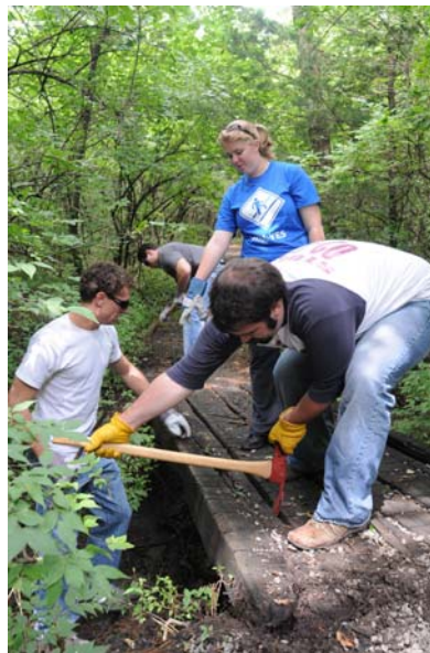
KU students worked hard during a day of service, pulling out the rotting ties of the Coralberry bridge.
